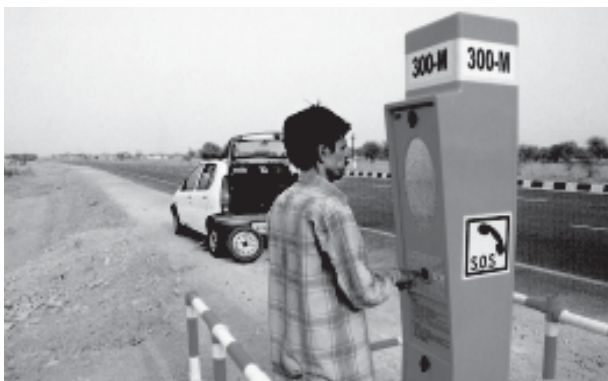
Fig.7.10 : Emergency call box on NH-8
